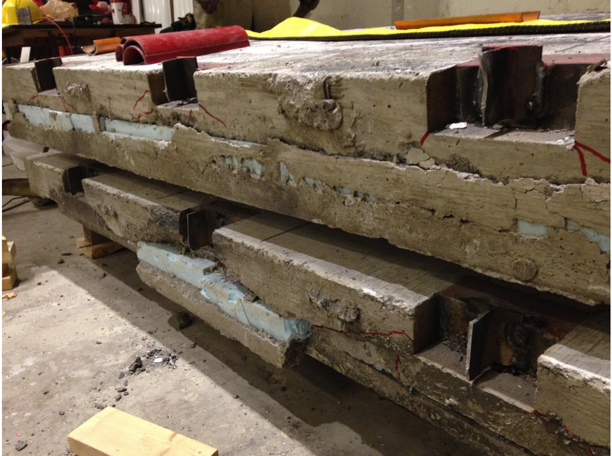
Figure 4.30 – NCTS-2 (Bottom) and NCTS-M (Top): Side-by-Side View of Upper Connection Damage
