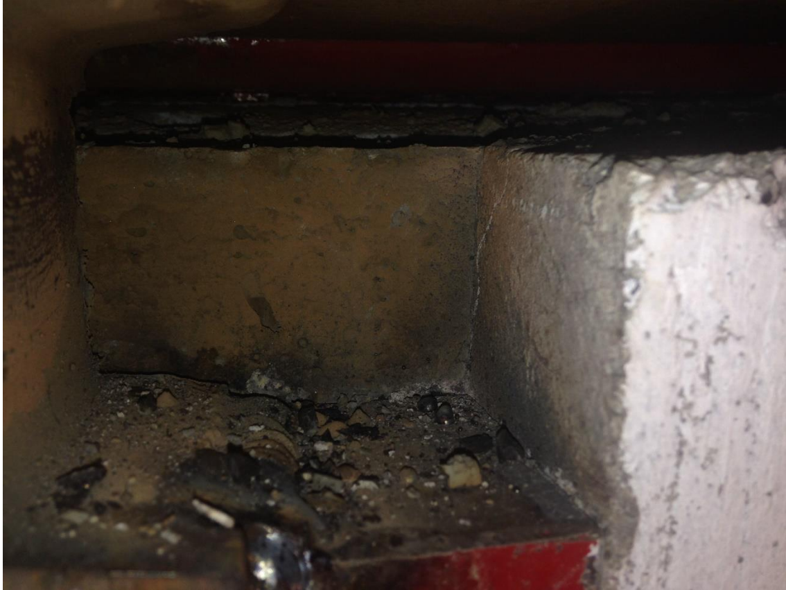
Figure 4.20 – NCTS-2: Typical Damage to Upper Connections and Shear Slip
