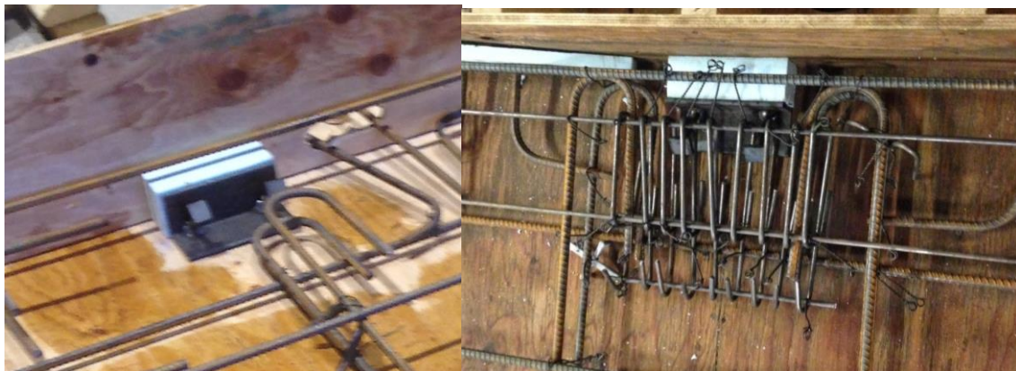
Figure 3.8 – Modified Support Reinforcement for NCTS-1 & NCTS-2 (Left) and NCTS-M (Right) Installed Prior to Casting
