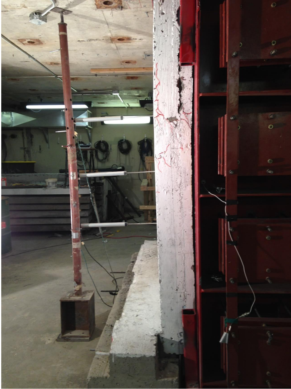
Figure 4.32 – NCTS-R: Side View with Flexural Cracks
