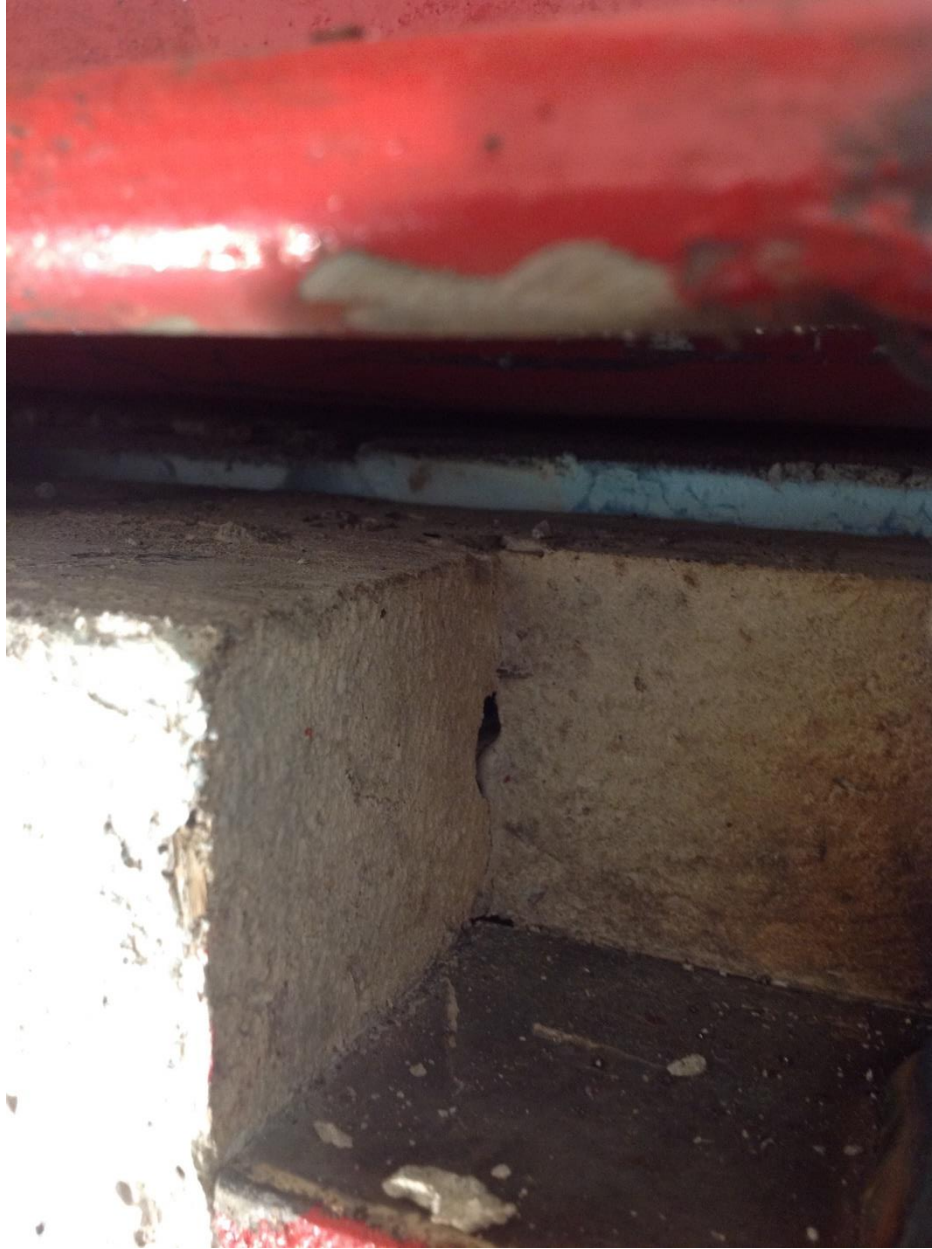
Figure 4.28 – NCTS-M: Cracks near the Upper Support and Shear Slippage between the Architectural and Structural Wythes following Test 3
