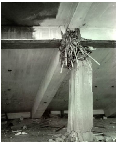
a) Reinforcement splice failure (Ref 1.)
