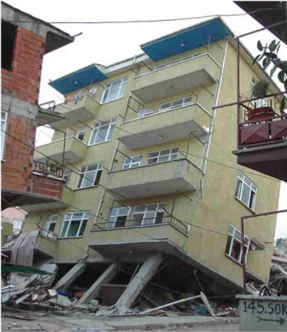
a) Soft storey collapse (Ref 9.)
