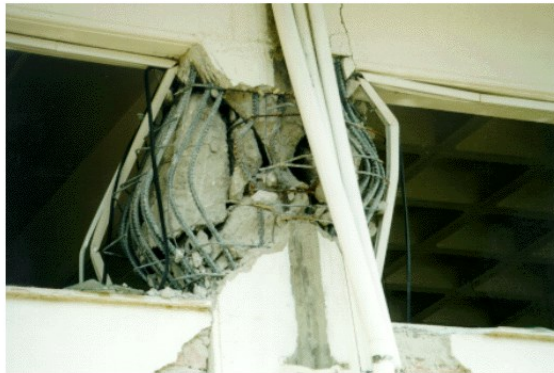
c) Shear failure in short column (Ref 3.)
