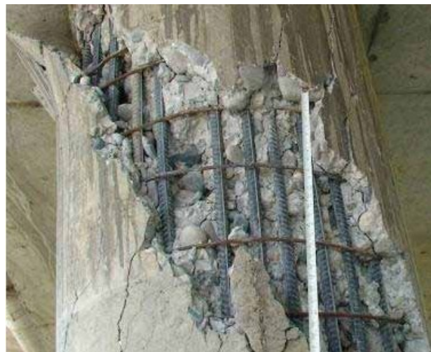
b) Column shear failure (Ref 2.)
