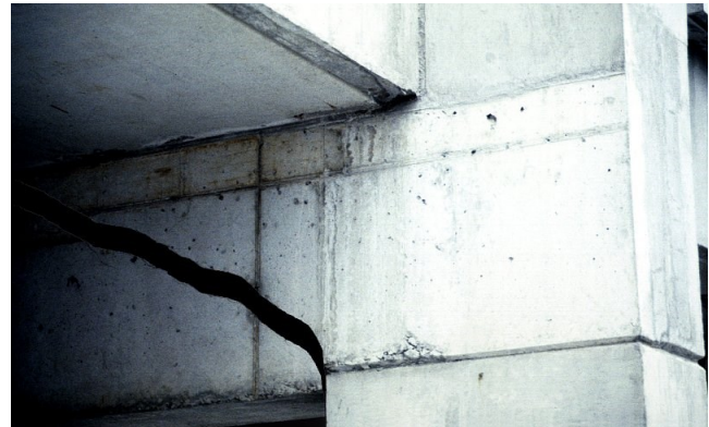
d) Beam diagonal tension failure (Ref 4.)
