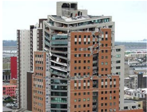
d) Torsional failure (Ref 12.)
