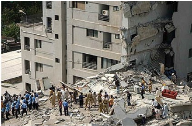
c) Damage associated with setback (Ref 11.)
