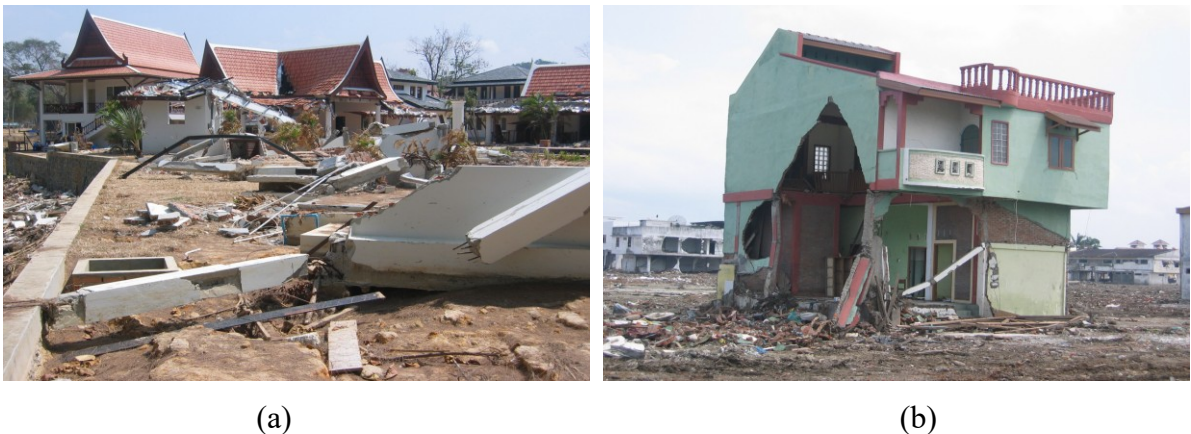
Figure 2.4 Tsunami-induced damage (Nistor et al., 2006): a) column failure in concrete frame, Khao Lak, Thailand; and b) punching failure of masonry infill walls, Banda Aceh, Indonesia
