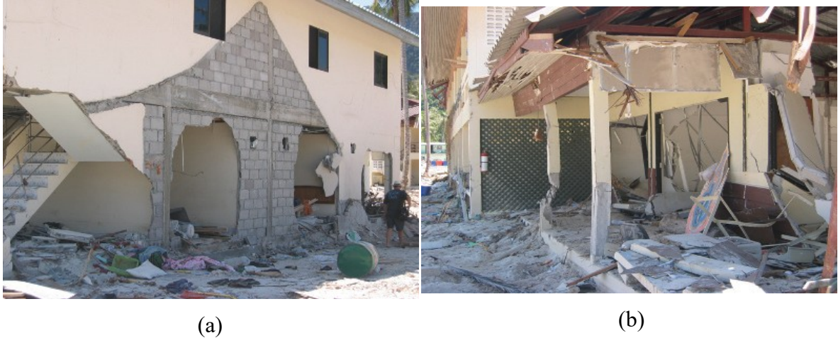
Figure 2.30 Damage to non-engineered reinforced concrete buildings, Phi Phi Island, Thailand (Saatcioglu et al., 2006): a) punching failure in masonry wall; and b) column failure due to debris impact
