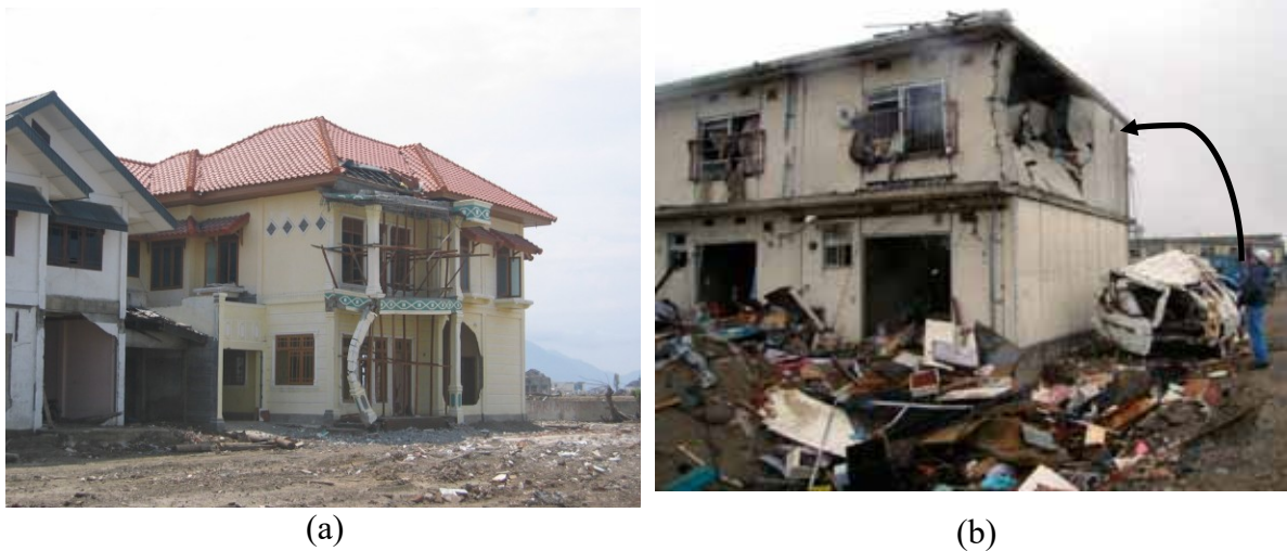
Figure 2.16 Damage to structural elements caused by tsunami-waterborne debris: a) column failure in reinforced concrete frame, Banda Aceh, Indonesia (Nistor et al., 2005); and b) impact failure of precast bearing wall apartment building in Yuriage, Natori, Japan (EERI, 2011)
