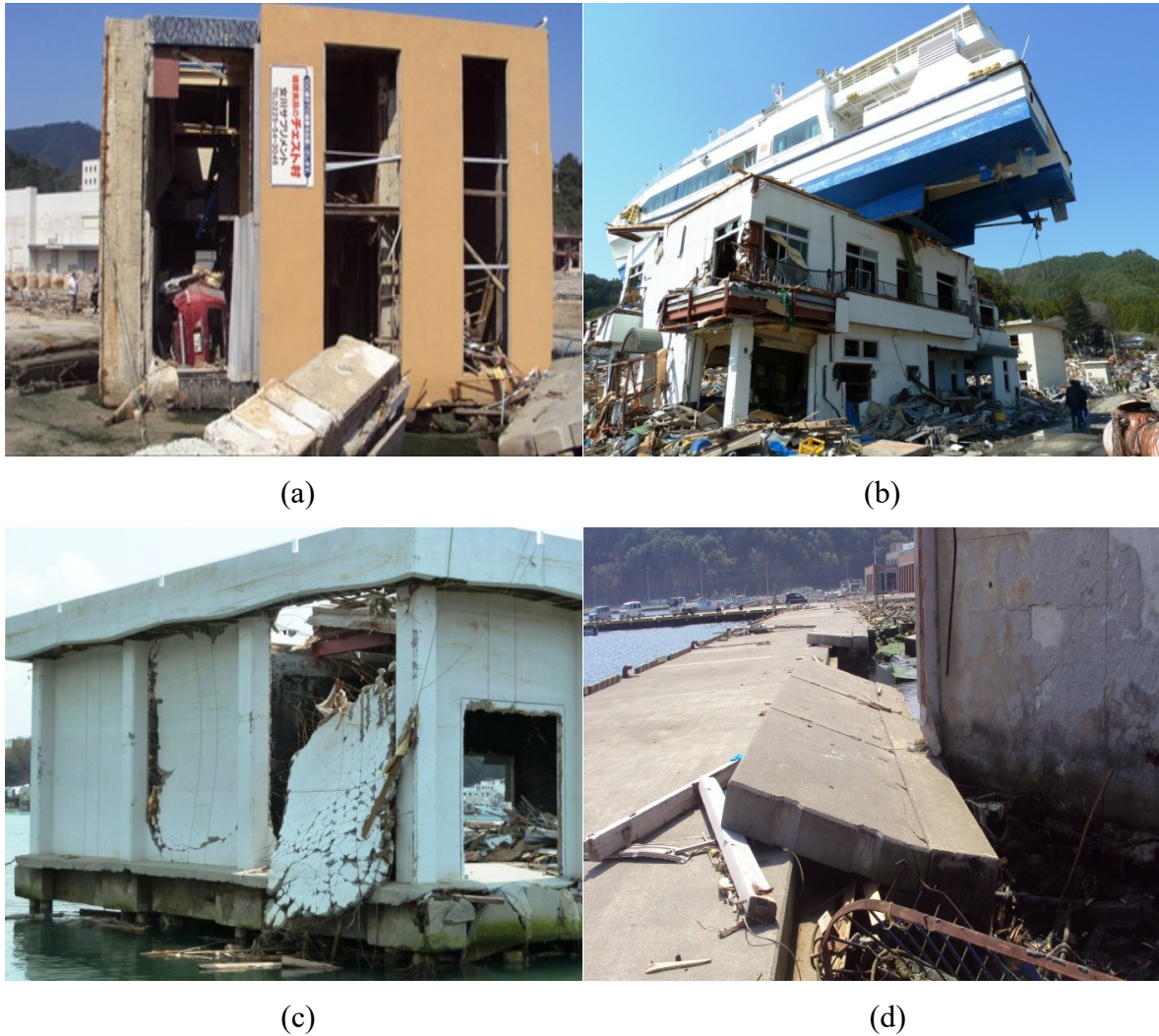
Figure 2.6 Impact of 2011 Japan Tsunami on residential and coastal structures (Nistor et al., 2012): a) steel structure overturned in Onagawa; b) impact loading from large vessel in Otsuchi; c) punching failure of fish storage building in Onagawa; and d) floating of concrete slabs in Onagawa
