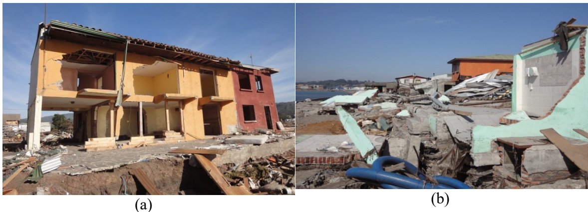
Figure 2.5 2010 Chile Tsunami damage (Palermo et al. 2013): a) punching failure of masonry infill walls and failure of columns in Pellhue; and b) widespread residential destruction in Talcahuano
