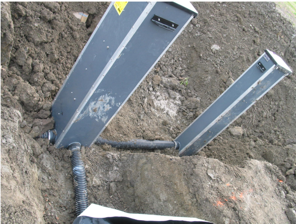
Figure 6: Pre-bioreactor control structure (left), bypass control structure (right), and connection to bioreactor (bottom) during installation.
