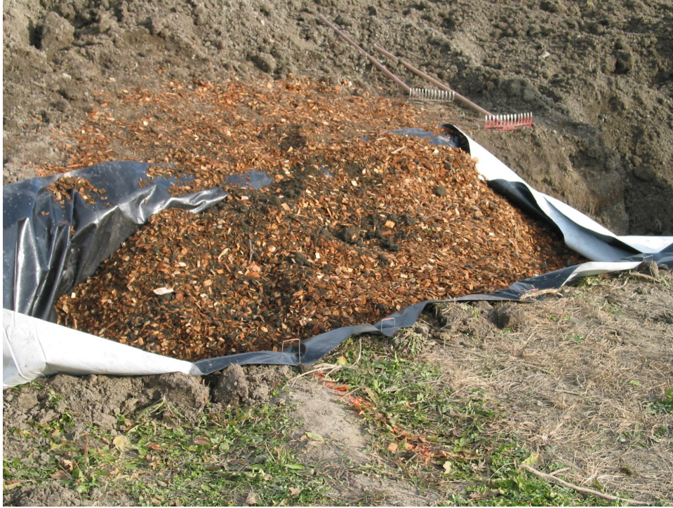
Figure 7: Woodchips added to a reactor bed during construction at Winchester field location.
