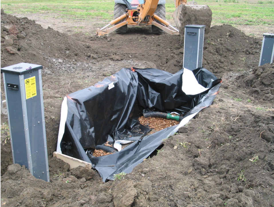
Figure 5: Bioreactor installation partway through construction. Pre-bioreactor (BBR) control structure and bypass control structures are shown in top-right; post-bioreactor (ABR) control structure is on bottom-left. Plastic wrap is shown partially installed as well as perforated input/output tiles on opposite ends of the reactor bed.
