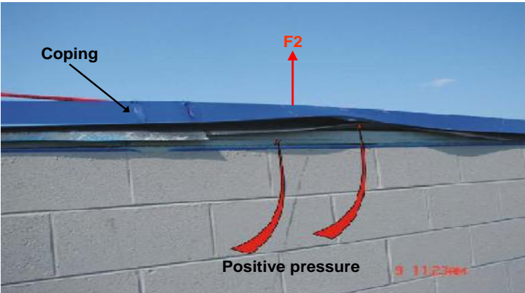
Figure 1.2 Severe deformation of the coping and cleat due to wind uplift forces (reproduced from Baskaran 2011)
