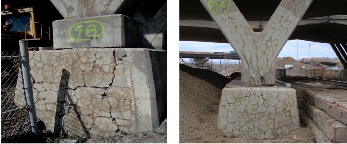
Figure 1.1: ASR map cracking on the reinforced concrete Y-shaped piers and massive concrete foundations of the Robert-Bourassa/Charest viaduct, Quebec, Canada (Sanchez et al., 2015)
