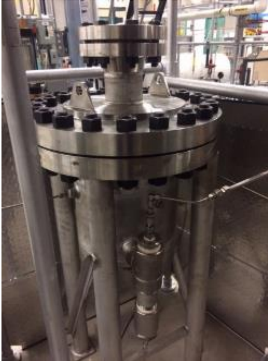
Figure A-2. Pressure vessel containing auger feeder
