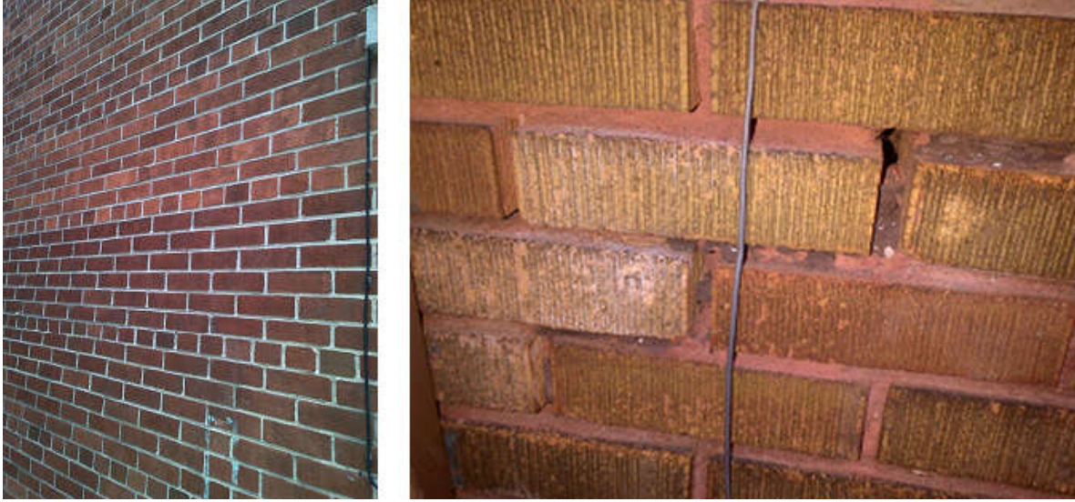
Figure 3-3: Masonry in good condition (left) and poor condition (right)
