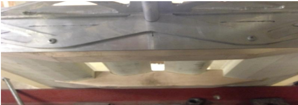
Figure 3.1.14 Bottom side of cross girders covered by small pieces of wood
