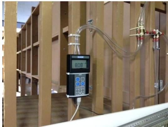
Figure 3.1.17 Wind speed controller
